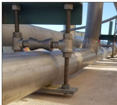
Picture 7 – Roller Pipe Support
