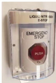
Picture 37 – Push Button E-Stop (Emergency Stop)
