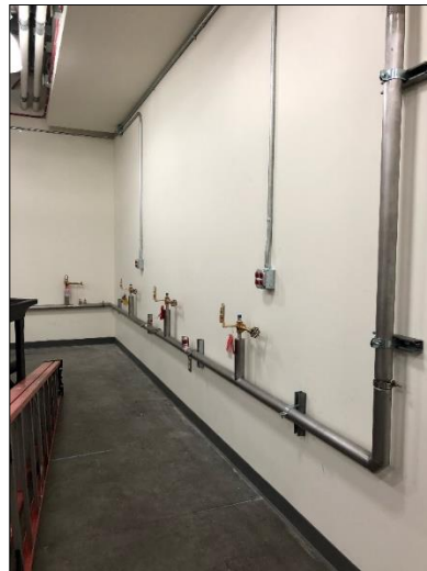
Picture 5 – Strut Pipe Clamp Support
