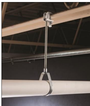
Picture 6 – Loop Hanger Pipe Support
