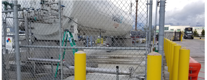
Hydrogen Extended Fill Line
