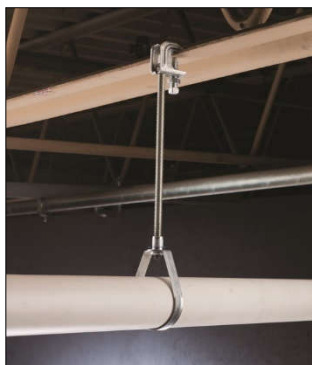
Picture 6 – Loop Hanger Pipe Support
