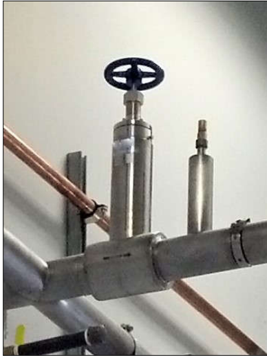
Picture 23 – T-Pattern Shut off Valve
