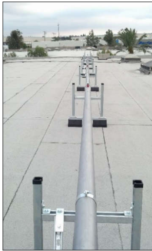
Picture 4 – Synthetic Roof Pipe Support
