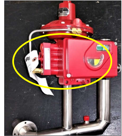
Picture 29 – Actuated Valve
