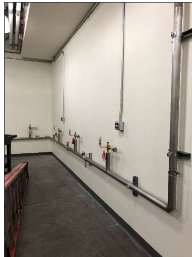
Picture 5 – Strut Pipe Clamp Support
