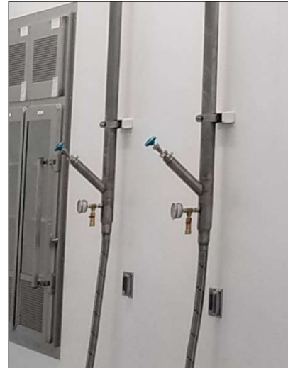
Picture 24 – Y-Pattern Shut off Valve
