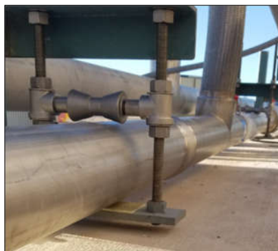
Picture 7 – Roller Pipe Support
