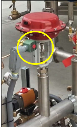
Picture 27 – Actuated Valve
